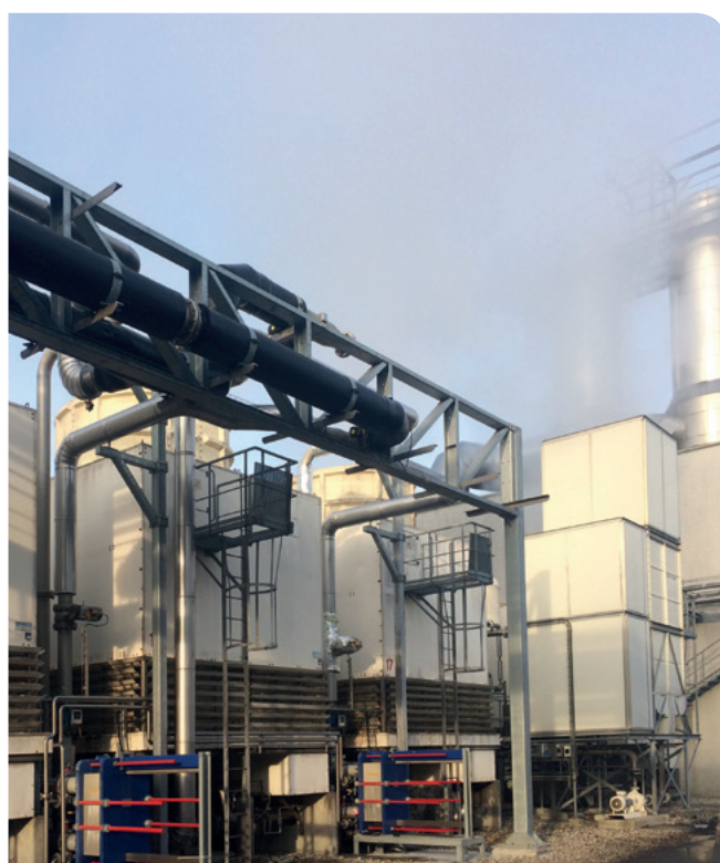
Existing cooling towers, which will, in the future, only be used as back-up if the district heating system cannot receive the surplus heat from the process at CP Kelco
