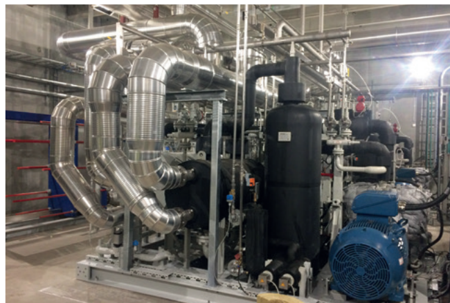
Heat pump where the flow temperature in the district heating system can be boosted from 72°C to 85°C if necessary.
